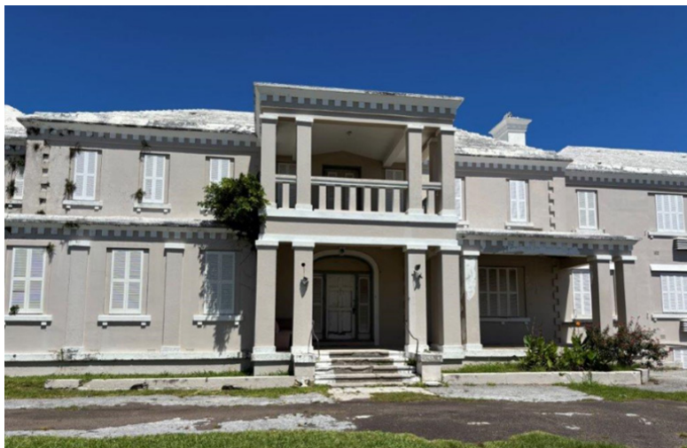
The overall condition of Loughlands today is one of abandonment and neglect. It's certainly not what a listed building should look like.
